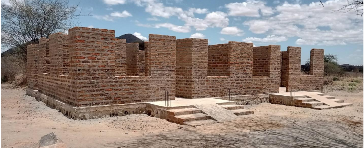
Photo #9: Construction of external and internal walls to the level of the rig beam
